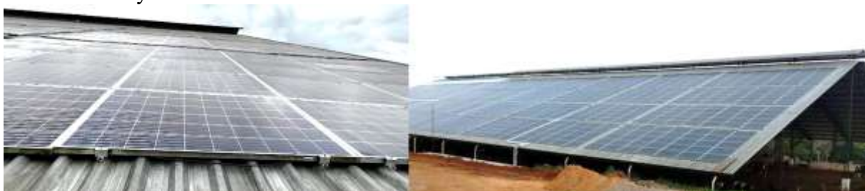
Figure 2 - Arrangement of photovoltaic panels on the roof of the Compost Barn (CB) under study.
